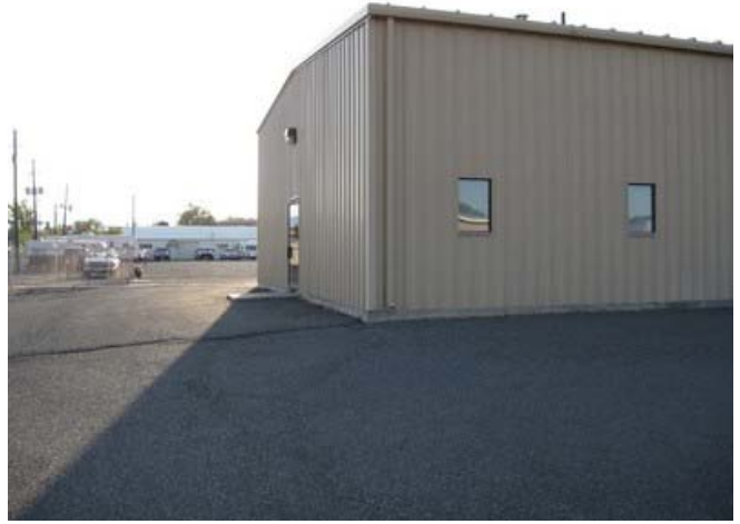
2: Location of asbestos-containing roof seam sealant (top of photograph).
