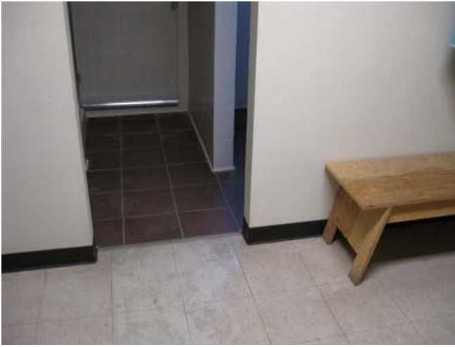
1: Asbestos-containing 12" x 12" floor tile and mastic.
