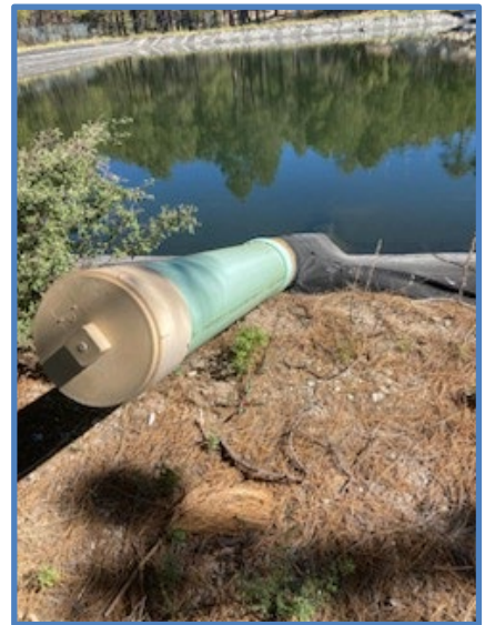
Existing Leak Detection Pipe
