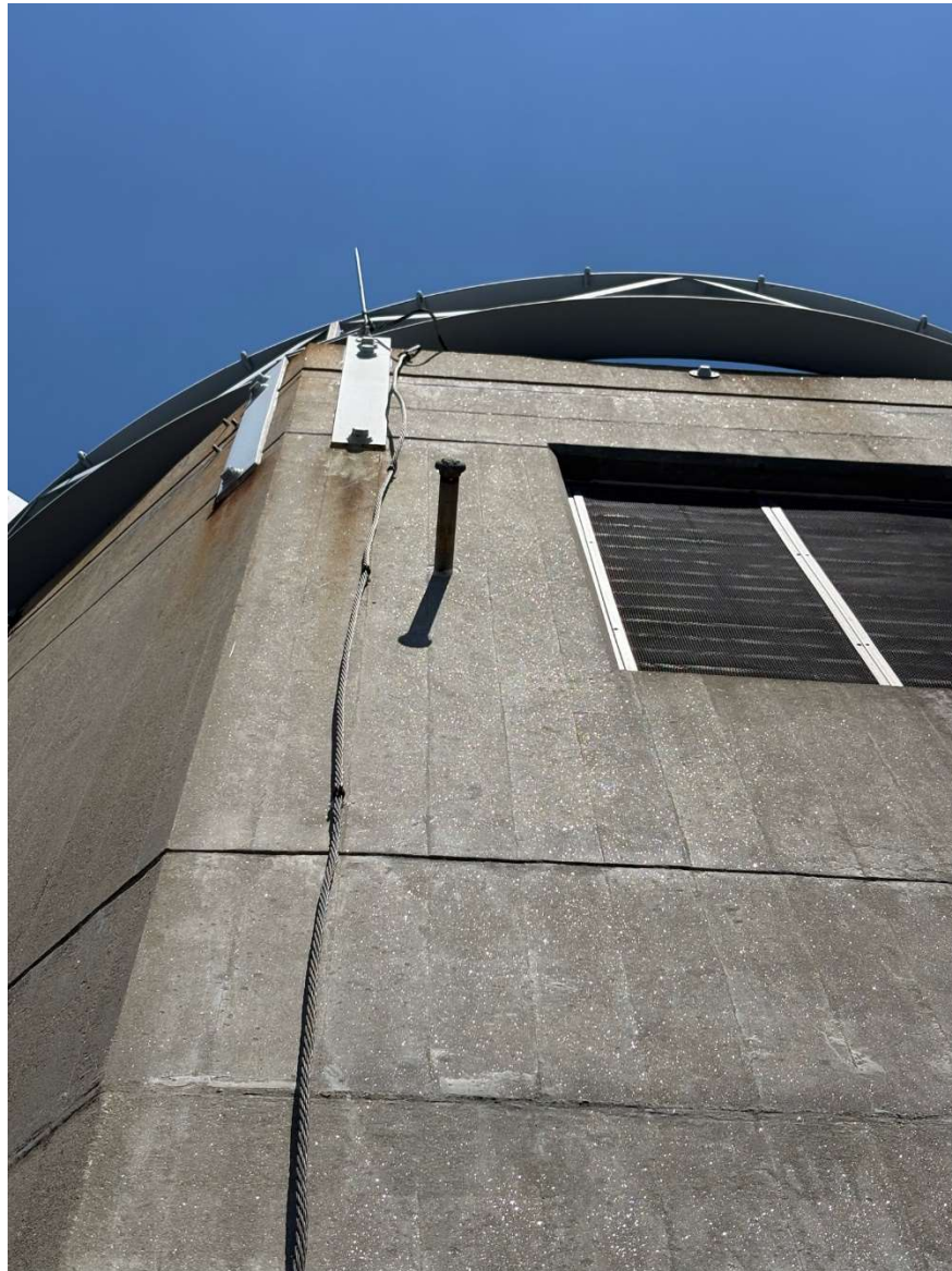
Colebrook River Lake Day Tank Vent Pipe, Located on the West Side of the Tower
