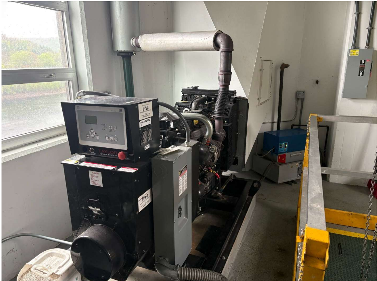
Colebrook River Lake Generator, Located One Floor Above Main Level
