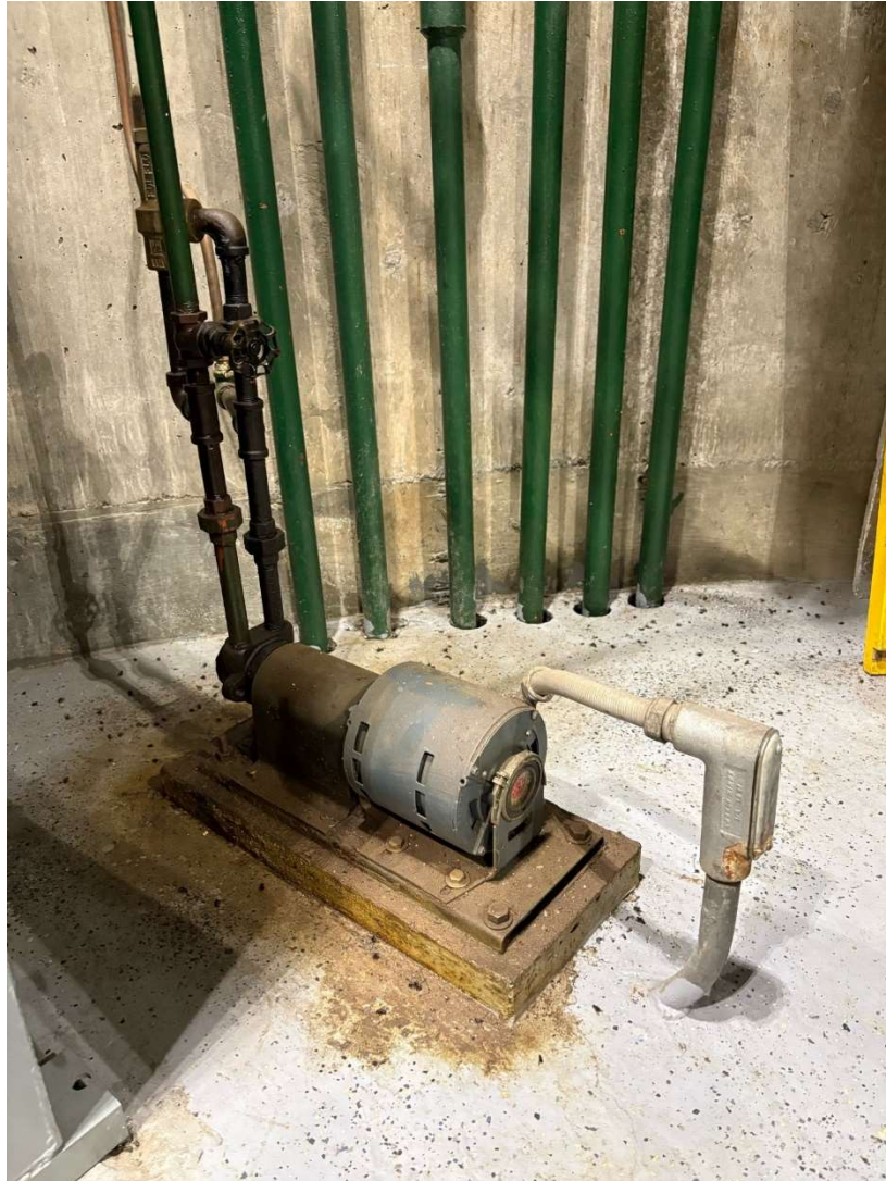
Colebrook River Lake Day Tank Transfer Pump, Located on Floor Below Main Level
