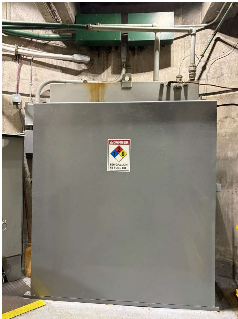
Colebrook River Lake Fuel Tank, Located on Floor Below Main Level
