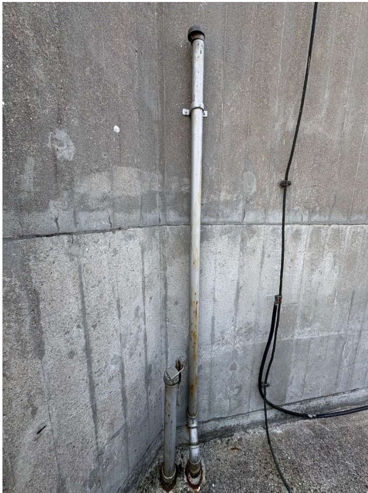
Colebrook River Lake Oil Tank Fill and Vent Pipe, Located on the East Side of the Tower
