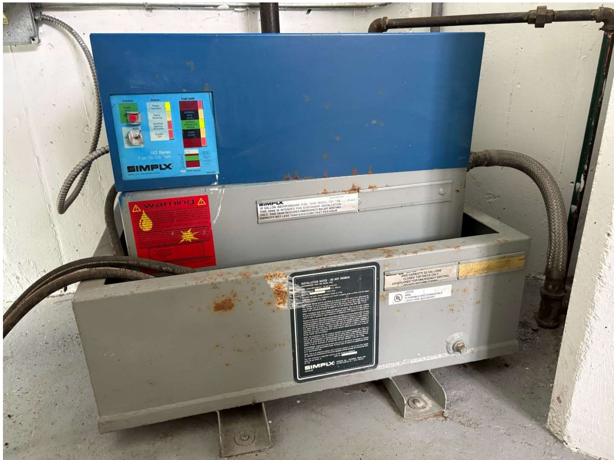
Colebrook River Lake Day Tank, Located on Floor Above Main Level
