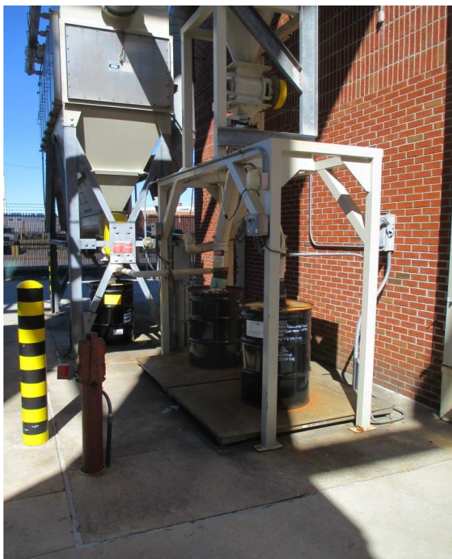
Photo 7: North facing view of blast debris collection equipment adjacent to the ASF.
