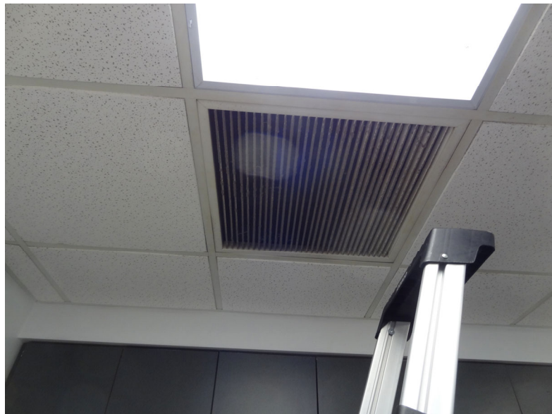
Photo 16: Typical view of a dirty HVAC diffuser observed in the building.
