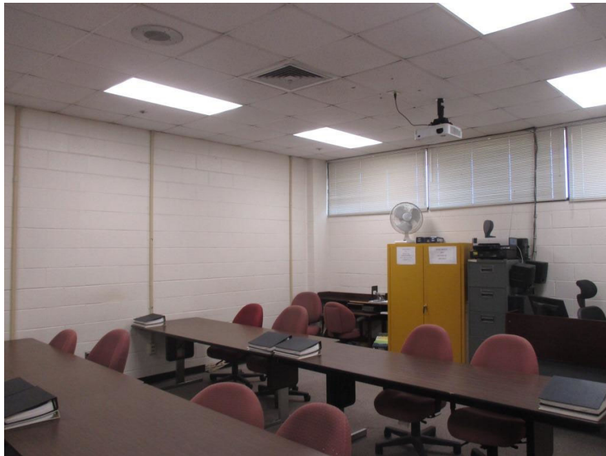
Photo 1: North facing view of the classroom #7. Sagging SACT and rusted SACT grid was observed in the original building.
