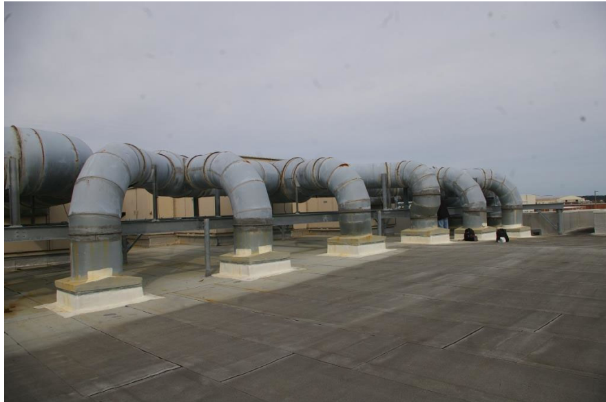
Photo 13: North facing view of the PMB roof area and ventilation equipment.
