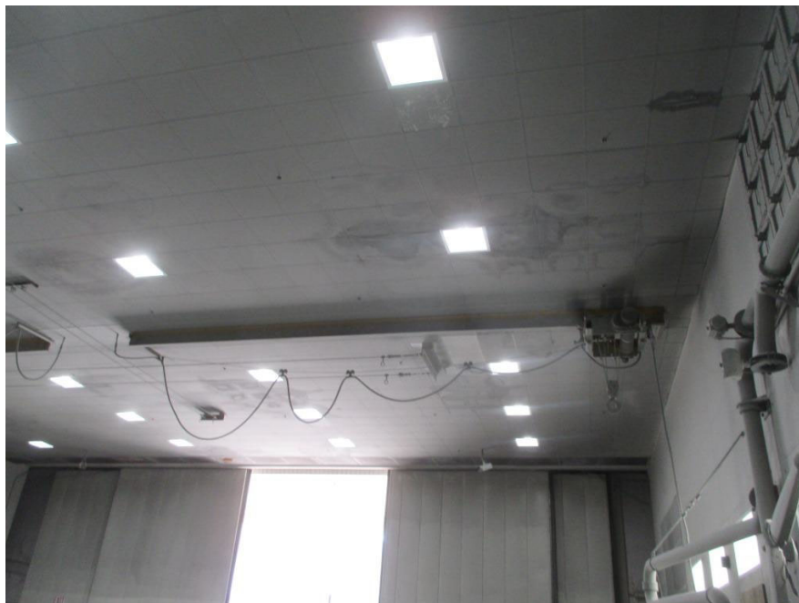
Photo 5: View of the SACT in the blasting room. The ceiling is assumed to be ACM until proven otherwise.
