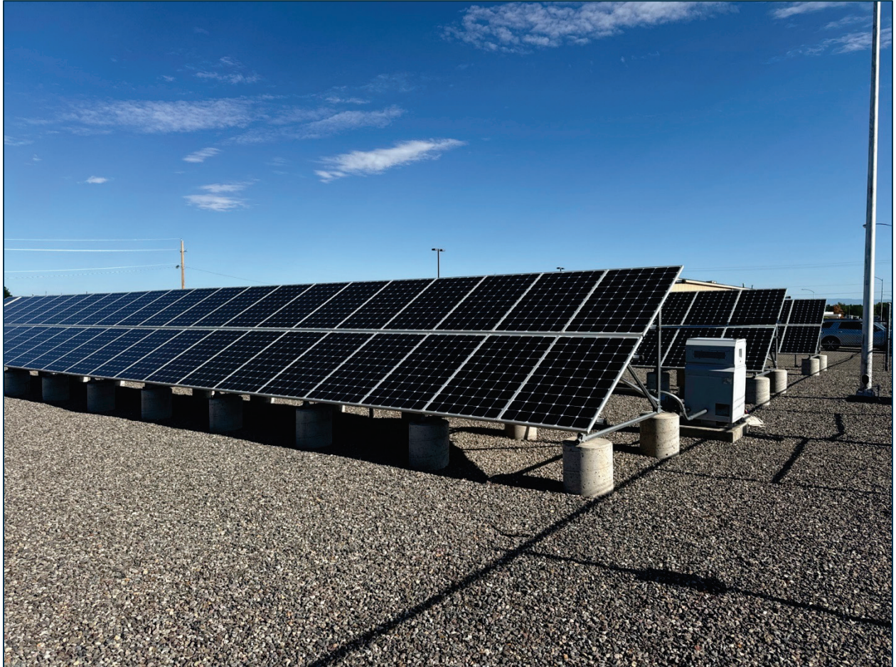
Figure 4: Uncompahgre site, showing the non-functional inverter
