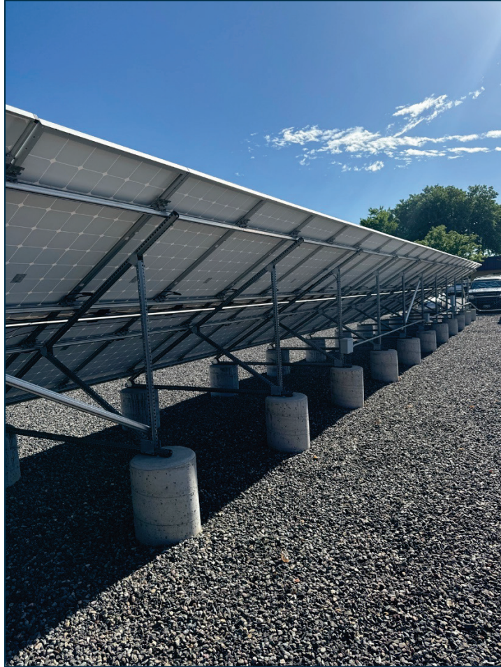
Figure 3: Wire management and mountings are all very good condition
