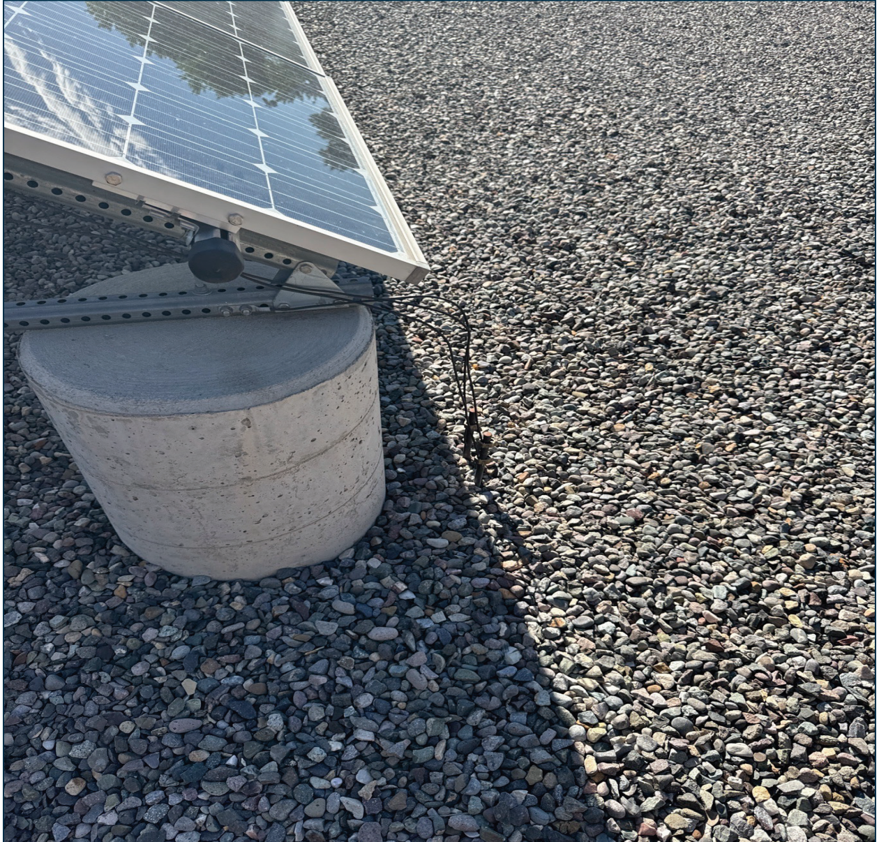
Figure 5: Typical grounding at Uncompahgre
