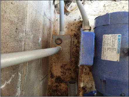
EXISTING ELECTRICAL CONNECTION
