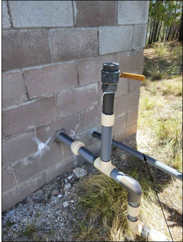
SUCTION SIDE OF PLUMBING
