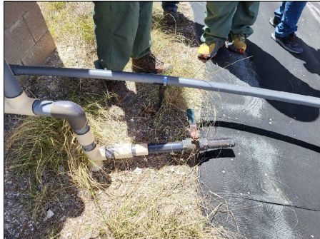
SUCTION SIDE OF PLUMBING
