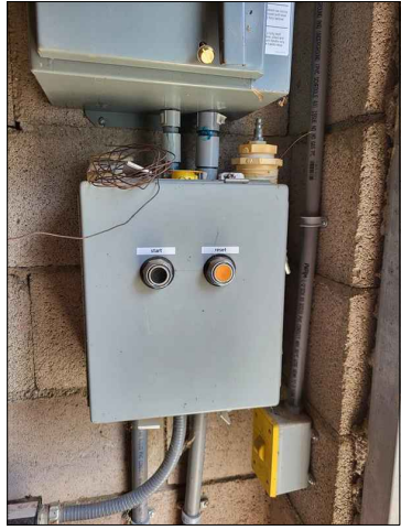
ELECTRICAL PANEL WITH MANUAL START AND RESET BUTTONS
