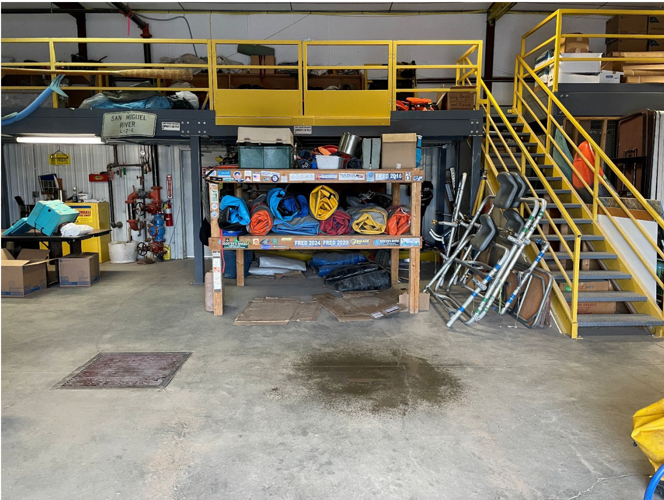
Roof leak – wet spot of floor is a roof leak.
