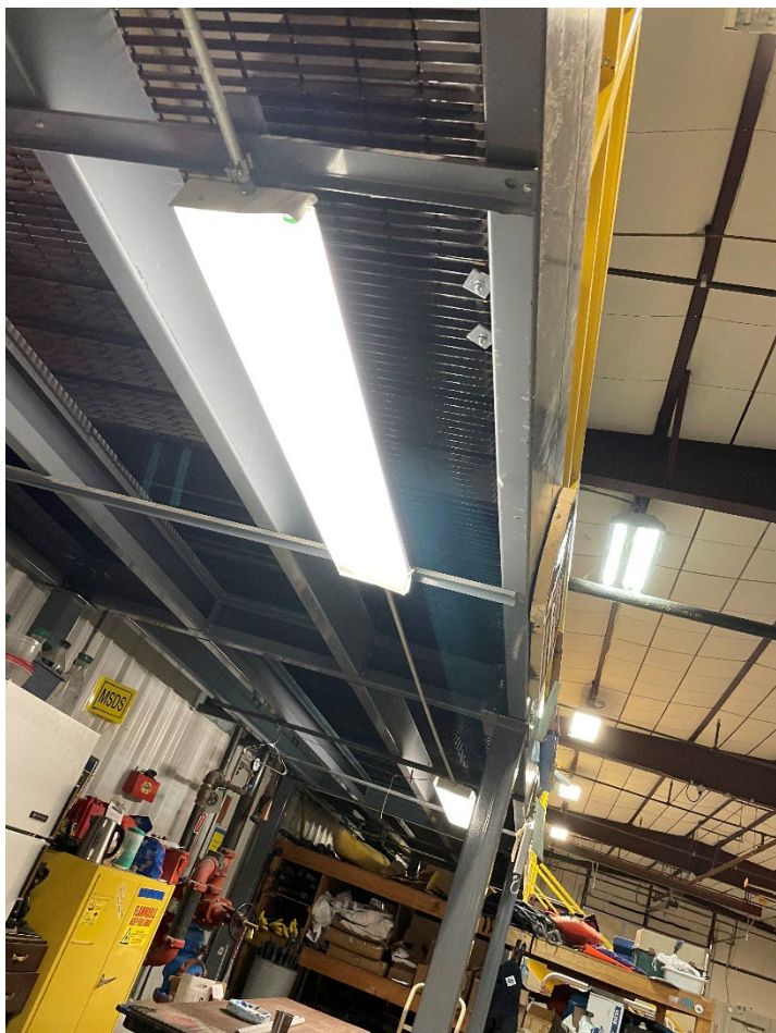
Typical warehouse luminaires – to be replaced.
