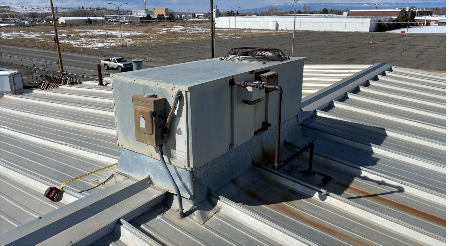
Rooftop HVAC unit – to be replaced.
