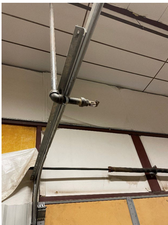
Warehouse sprinkler head near garage door track
