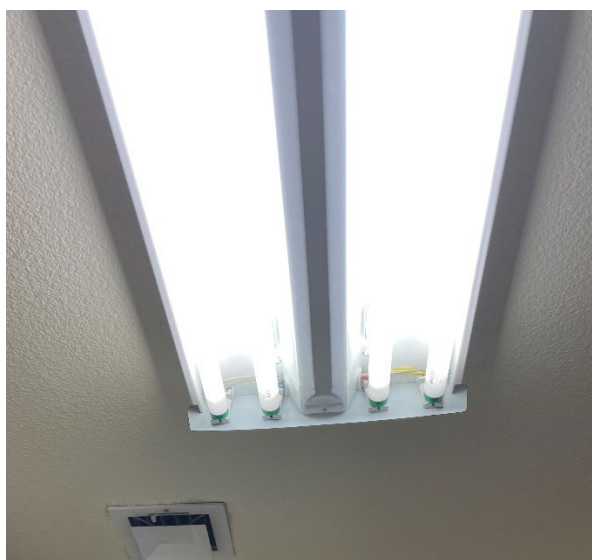
Typical office and bathroom luminaires – to be replaced.
