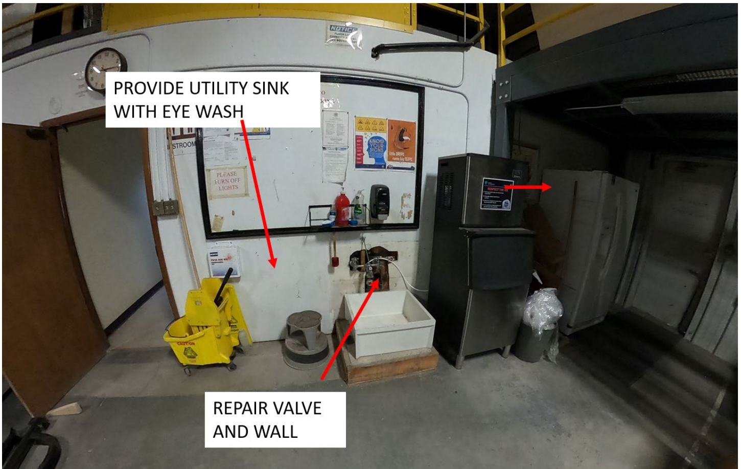
Warehouse – proposed utility sink, eye wash station, and plumbing repair.
