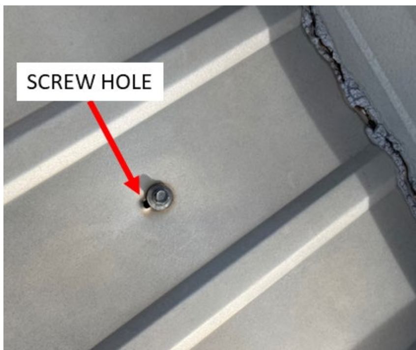
Screw holes in warehouse roof.
