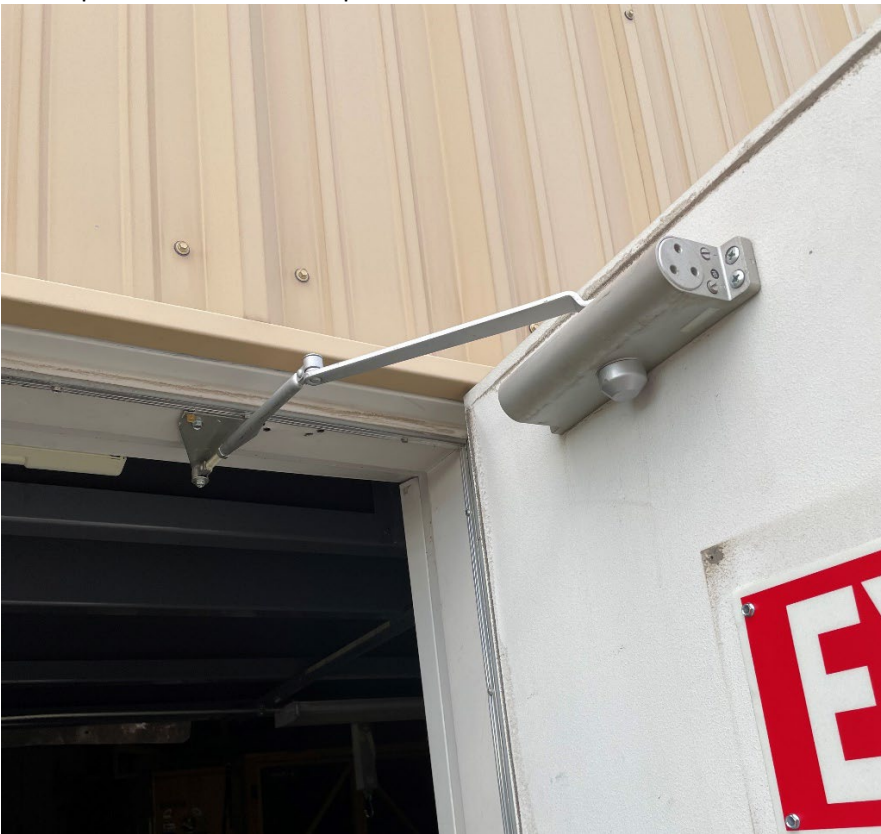
Warehouse Door Closer – to be replaced
