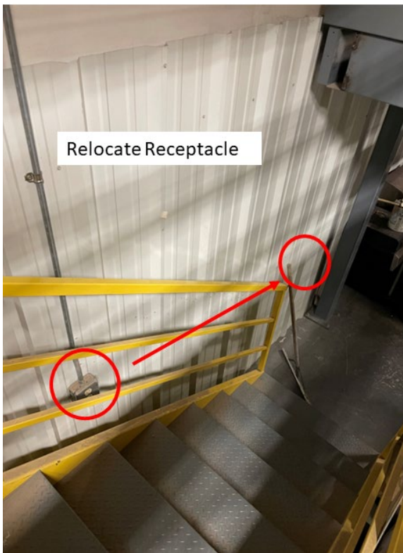
Electric outlet to be relocated.
