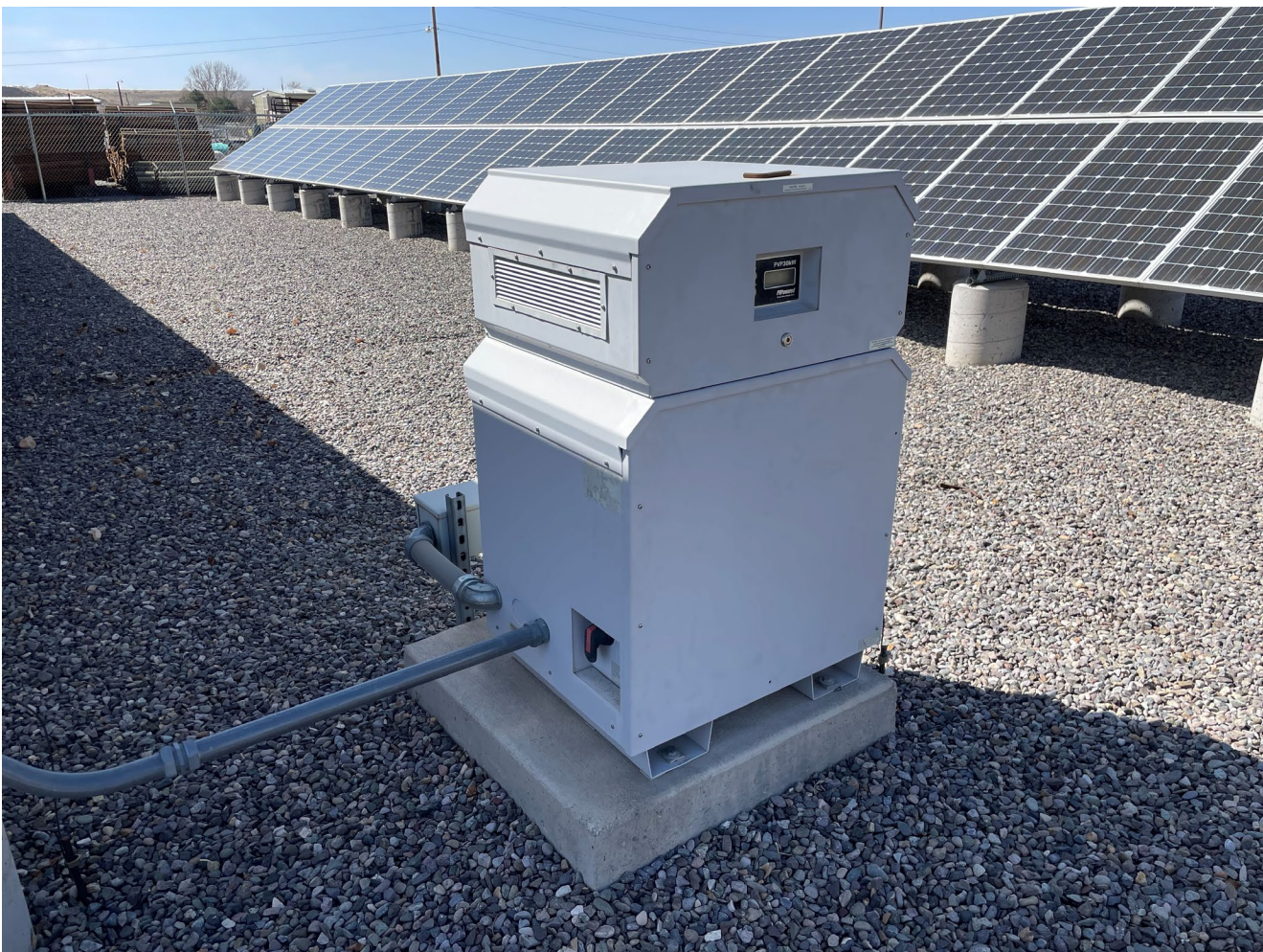
Photovoltaic Inverter – to be replaced.
