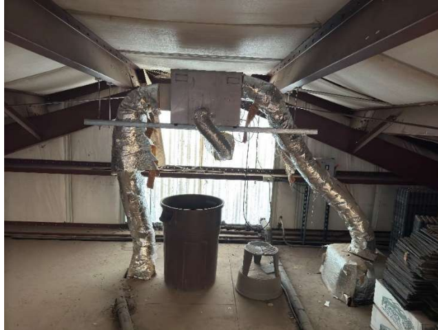
Figure 3: Old dehumidifier equipment on top of walk-in cooler, ducts, and electrical connection in the back wall – to be removed.
