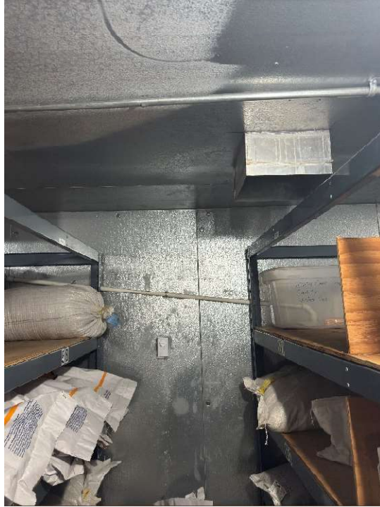
Figure 5: Inside of the cooler where vent and old humidistat are located.
