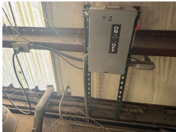
Figure 4: 240V electrical outlet available.
