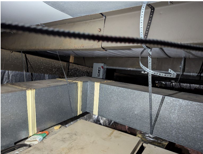
Figure 2: AIR HANDLER DISCONNECT.
