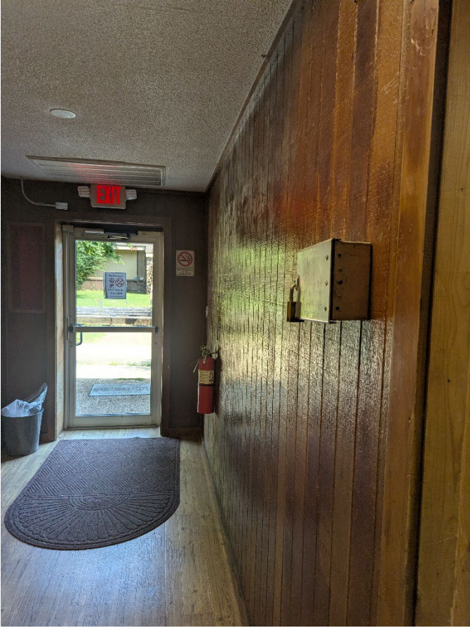
Figure 12: THERMOSTAT LOCK BOX.
