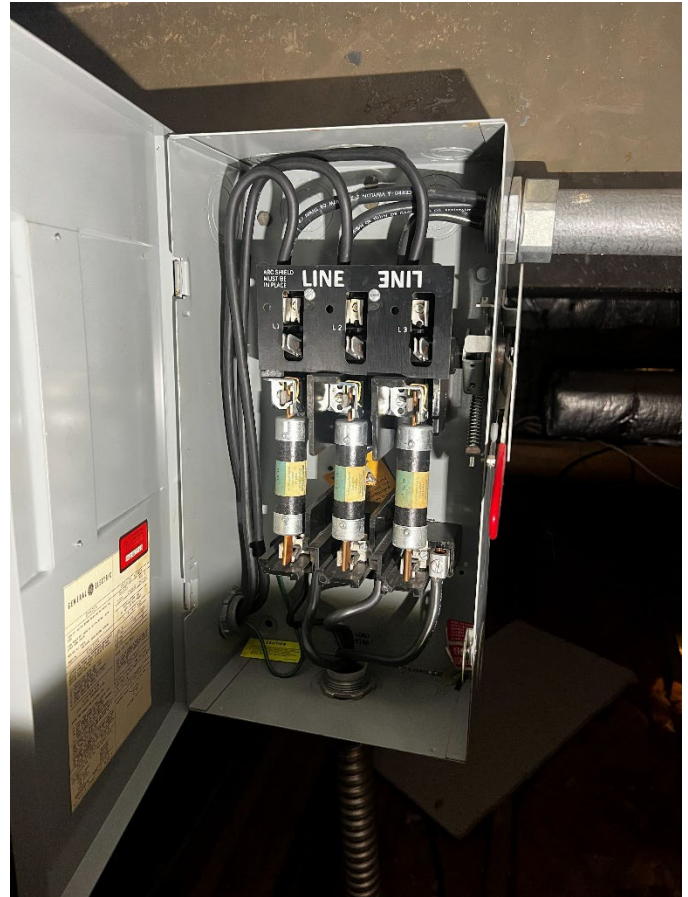
Figure 3: AIR HANDLER DISCONNECT.
