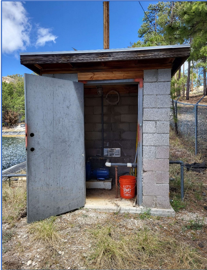
Palisades Lagoon Pumphouse
