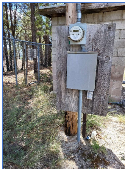
Existing Electrical Meter and Panel with Duplex Receptacle
