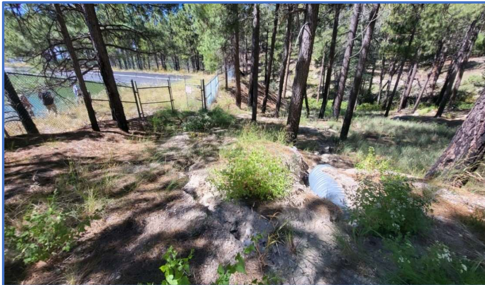
Eroded Service Access Road with Exposed Culvert & Erosion (taken 9/12/2024)
